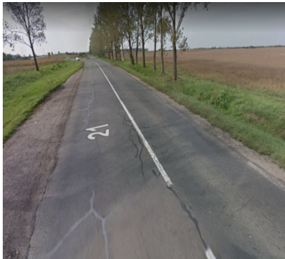
Figure 1. Separate segment of the existing variant of the section Ruma- Irig, where it is possible to change the horizontal signalization
