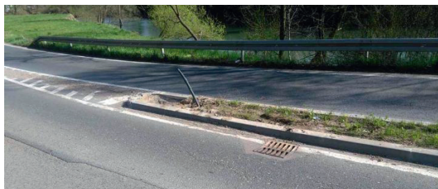
Picture 6. Condition on the subject spot from 2016 (4 March 2016)
