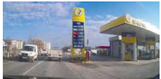
Figure 6. Unprotected steel structure of the gas station
