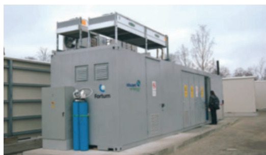
Figure 3. Hydrogen production plant (electrolyzer)
